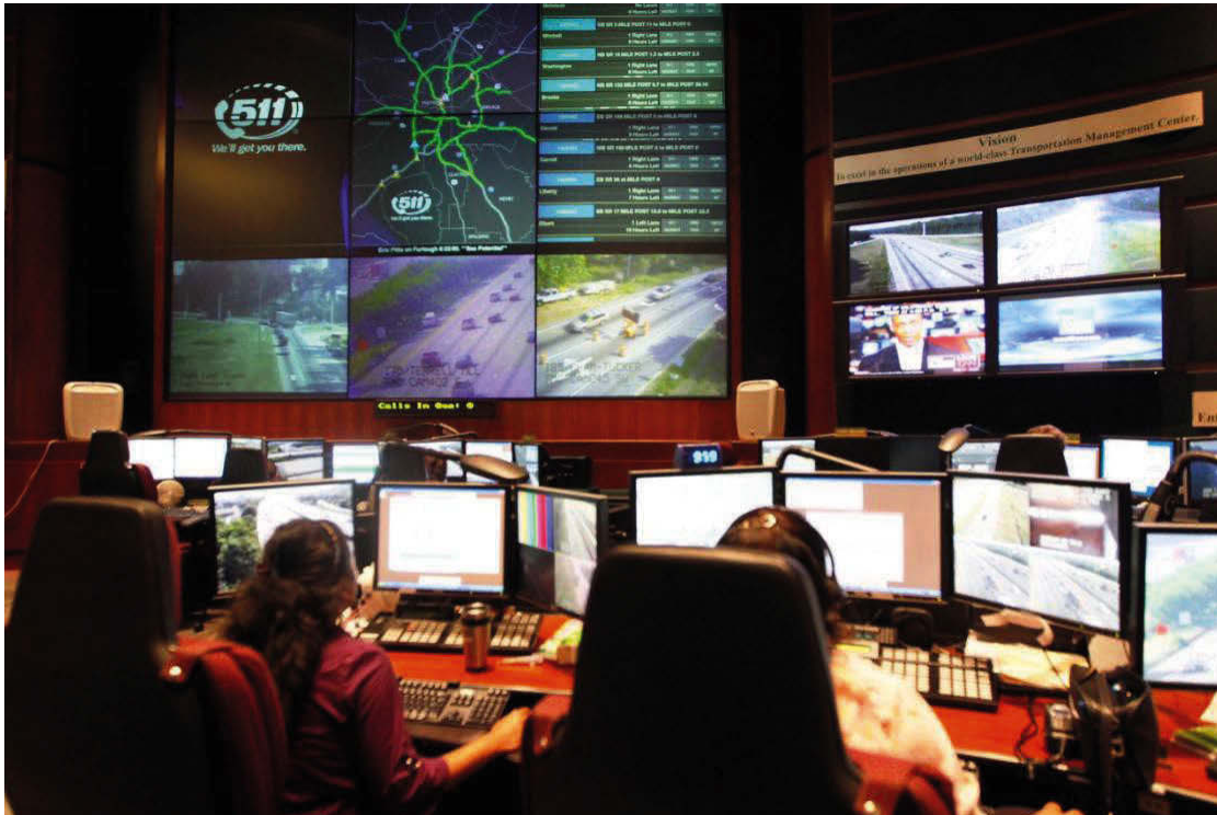
Figure 55 Georgia Department of Transportation Traffic Management Center
